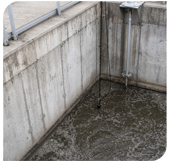
A VARiON sensor was installed in the anoxic basin to continuously monitor ammonium and nitrate during the trial.
